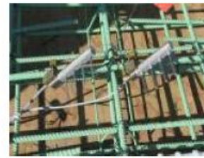
Concrete humidity and corrosion sensors
