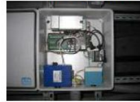
Vibrating wire and temperature sensors datalogger
